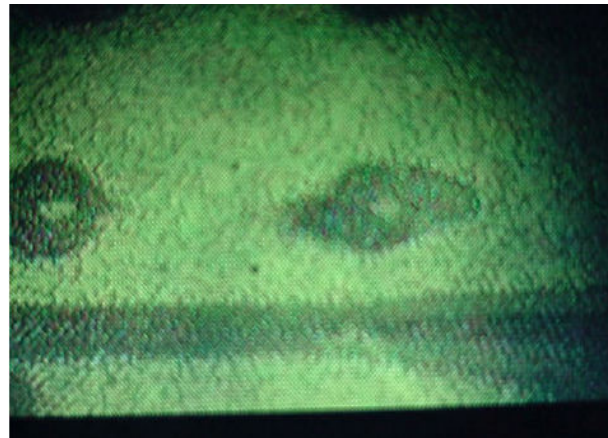
Lower row S-4R cracks as depicted by an emerging NDT method - external MOI.
